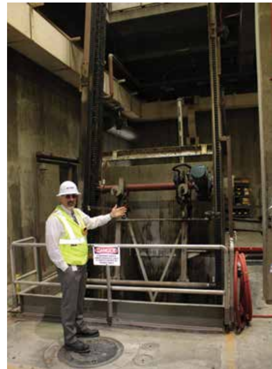
One of the barscreens which remove 'solid' material from waste water.
